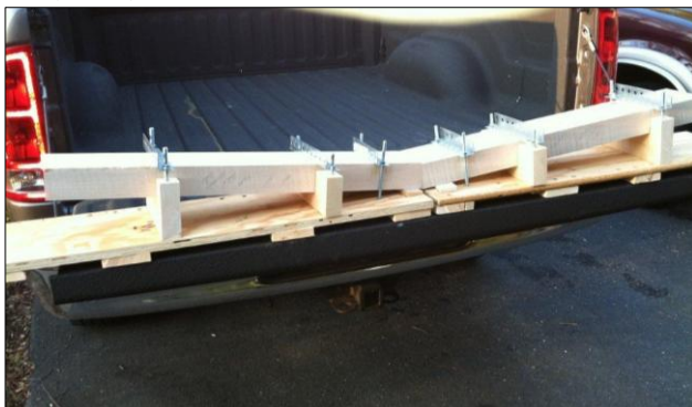
This will be the front header piece when completed. The photos show all of the pieces to be cut. Note
