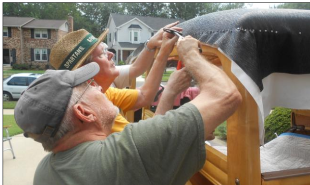
Nearly finished! Bill Selley, Dave Westrate and Wayne Chadderton (hidden) put the final tacks in above the left quarter panel.
