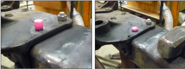
With the bucking bar in firmly in place, the rivet was heated cherry red and then peened over using a four pound hammer.
