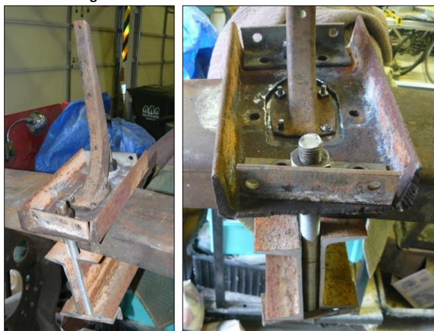
The bucking bar was installed and the running board support arm bolted in place. In the right photo one rivet has already been installed and another is ready for forming.
