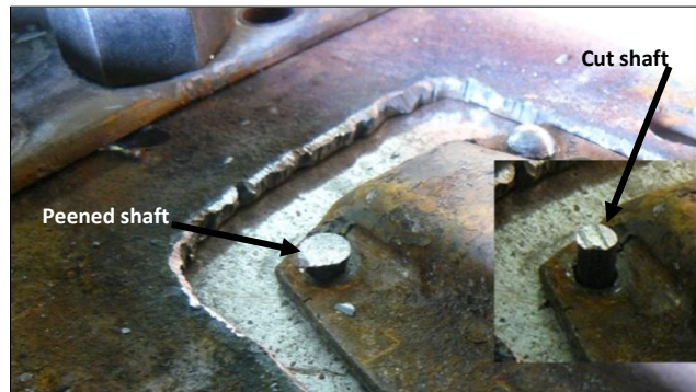
The picture above shows the rivet shaft has been peened over. The inset shows the amount of shaft protruding before being peened over.
