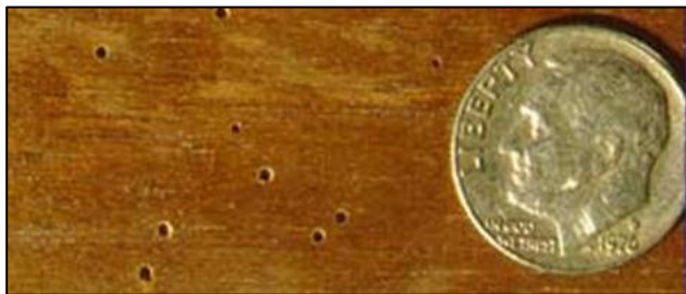
This is what Powder Post Beetle damage looks like. Beneath the surface is extensive unseen damage.
