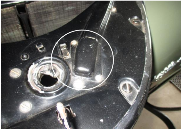
Early cover over only the cable end.
