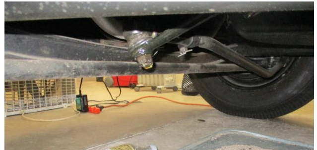
This view from the left side of the late car shows the drag link mounted on top of the replacement late steering arm.
