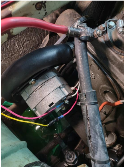
Modern alternator now replaces bad generator that failed
